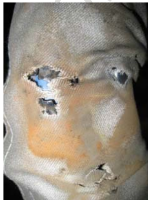
Fig. 2.2.3 (b) Damage on the cable protective sleeve
