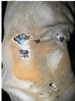
Fig. 1.2.5 (b) Damage on the cable protective sleeve
